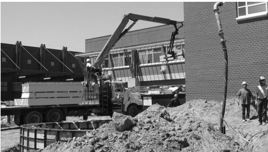
Construction work on the new Bruce Randolph Middle School, 3955 Steele Street, continued throughout the summer. Randolph is one of four new schools that will debut later this month.
